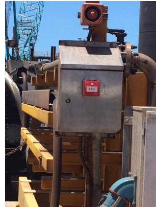
Figure 3: Northern alarm point
