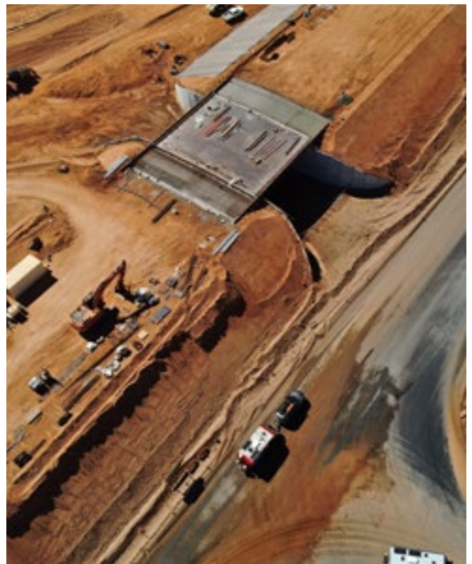
Progress on the roads and intersection upgrades with the underpass complete and bridges connected, June 2025.
