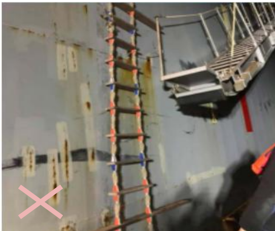
Non-compliant combination ladder arrangement
