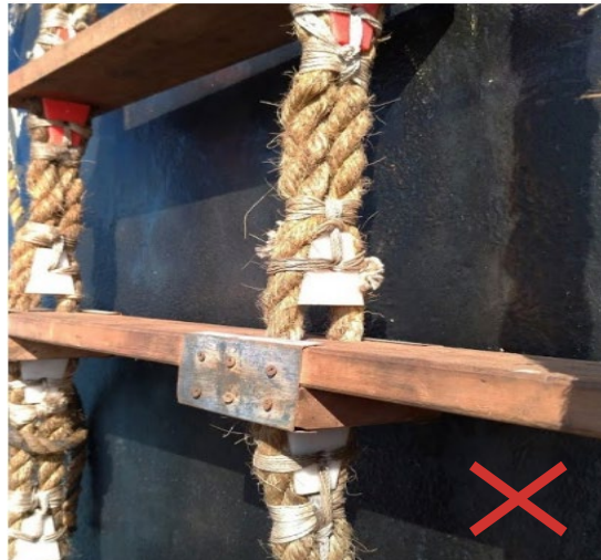
Spreader not made from a single piece of wood
